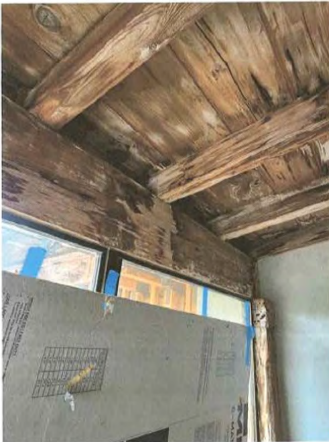
PHOTO 7 - West Balcony looking at roof framing with corner post in two pieces, without a connection
