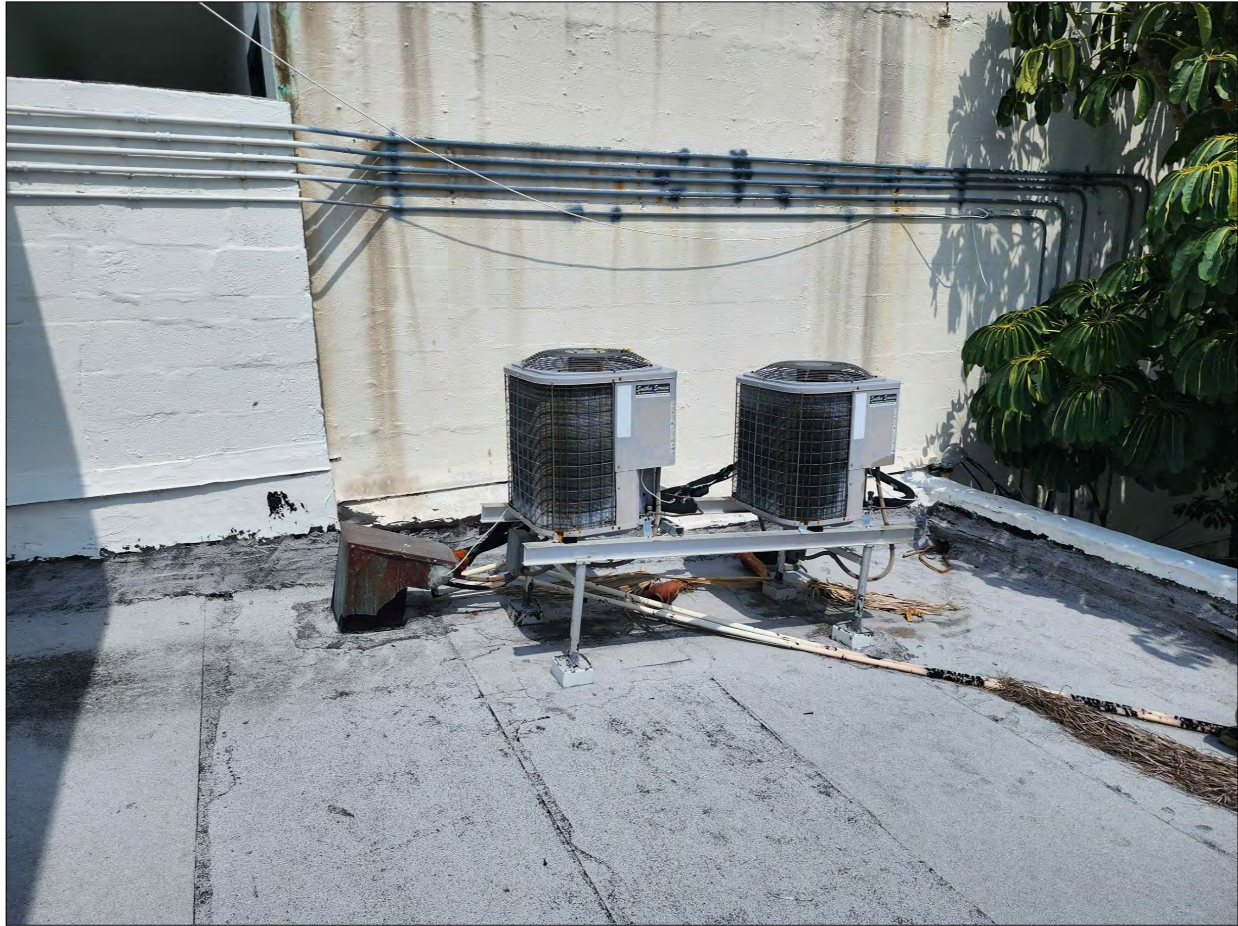
ROOF TOP AC UNITS
