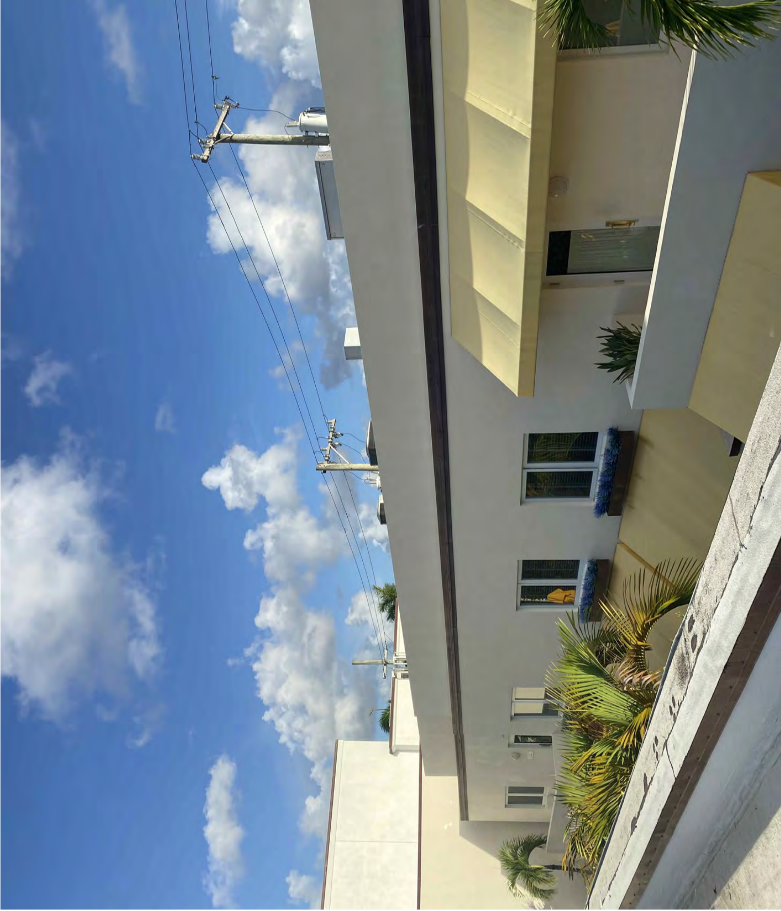
Equipment Screen Wall
