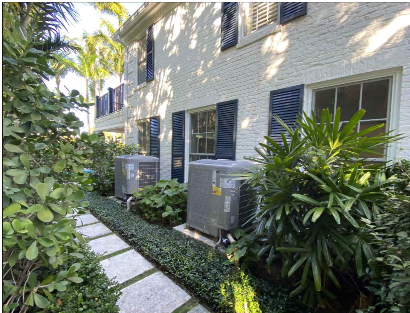
Ⓓ WEST SIDE YARD A/C EQUIPMENT
