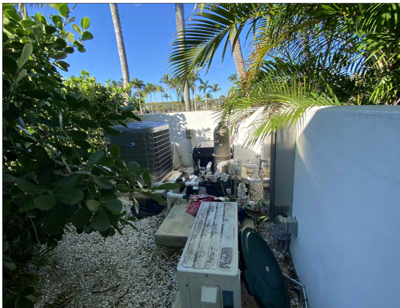
Ⓔ EXISTING POOL EQUIPMENT
