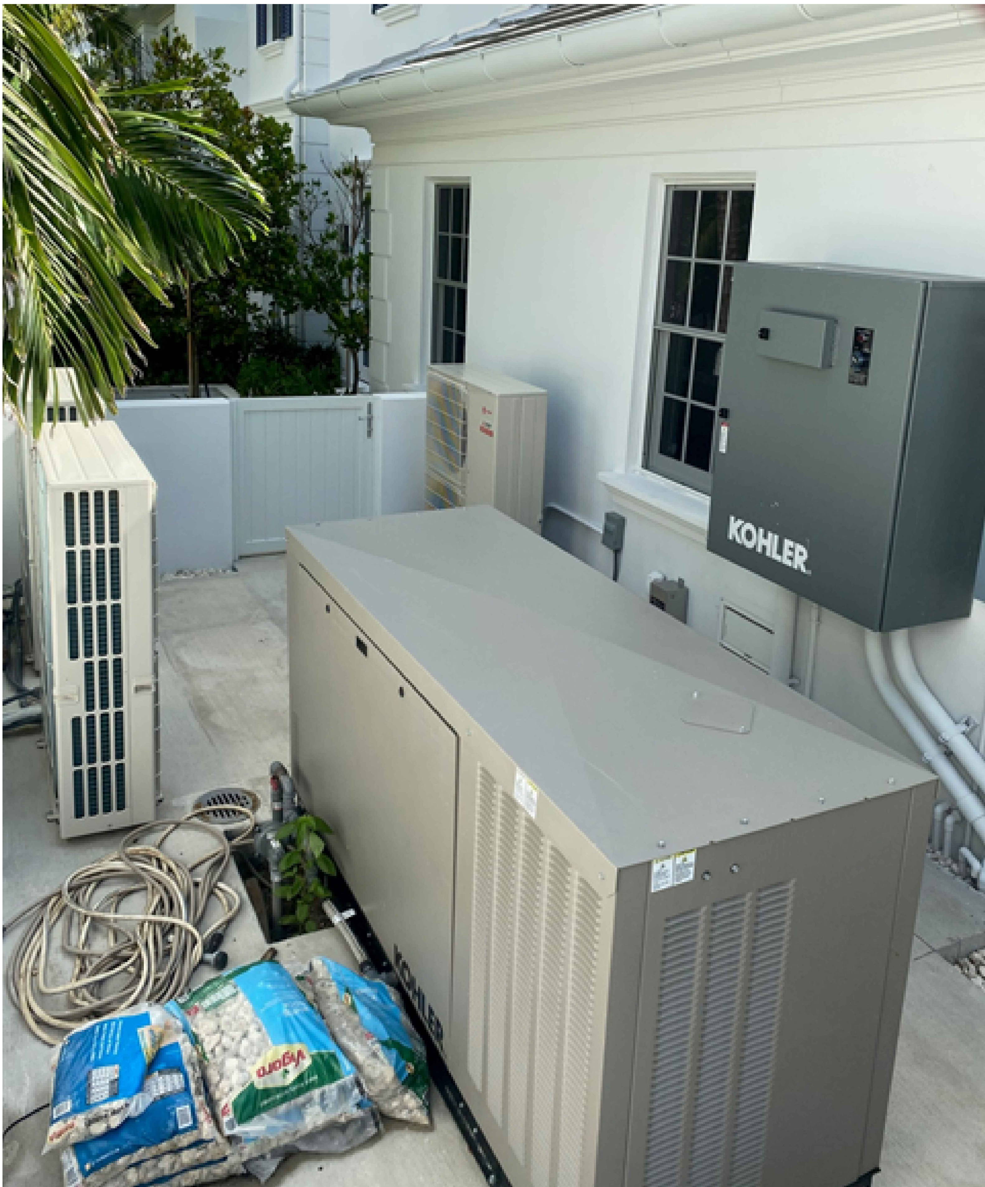
310 Clarke Avenue (Western Yard Equipment Area)
