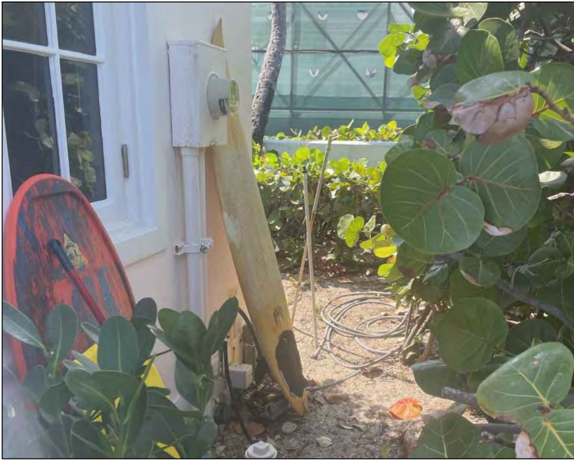
VIEW H - EXISTING METER AT NORTH ELEVATION
