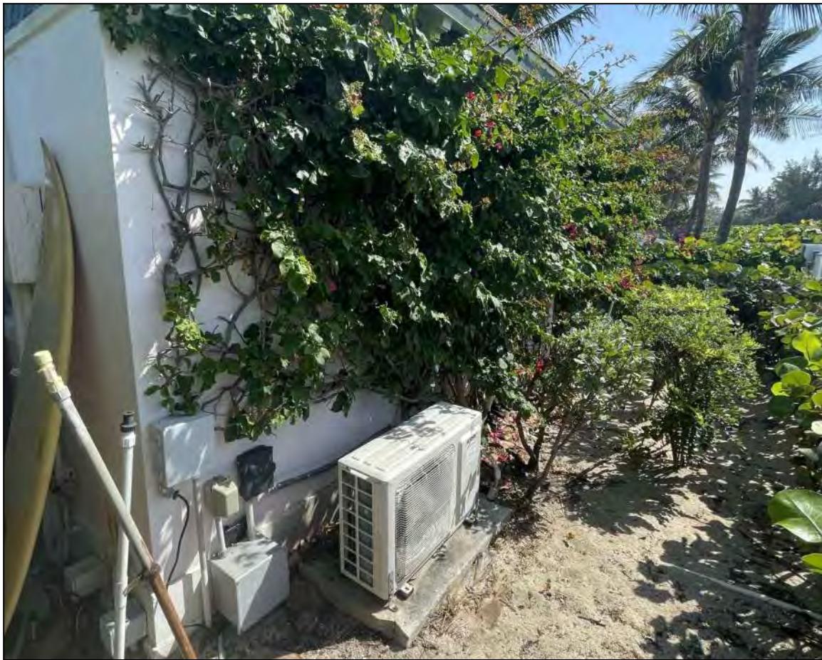
VIEW D - EXISTING EQUIPMENT AT WEST ELEVATION
