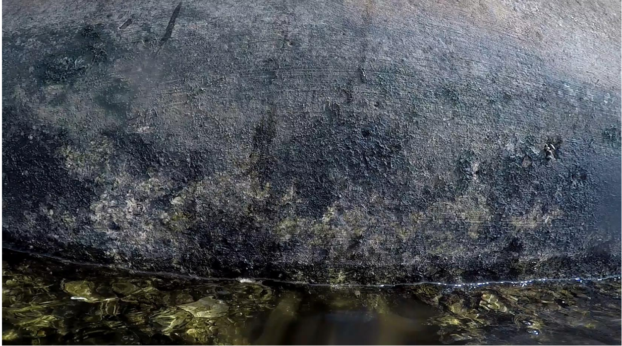
Figure 3.4: Sta 2+90. Typical bulkhead face transition from exposed concrete to the concrete covered in marine growth within in the intertidal zone.
