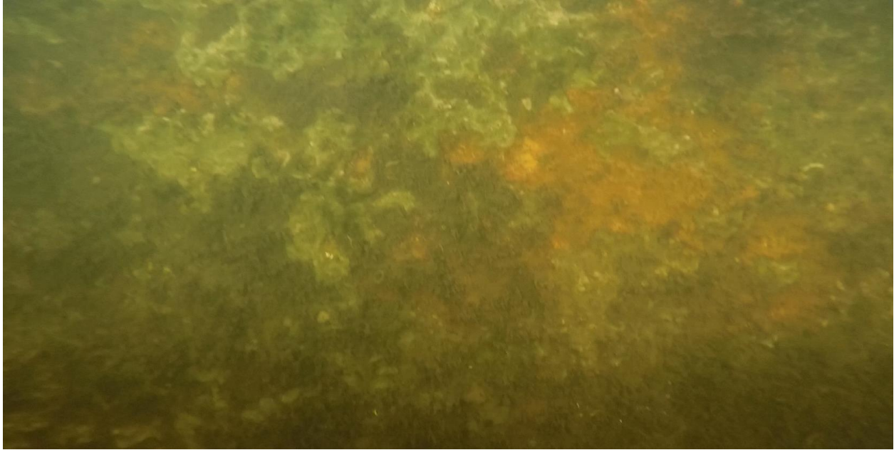
Figure 3.6: Sta 3+30. Infrequent rust coloration of marine growth suggestion corrosion within the bulkhead.
