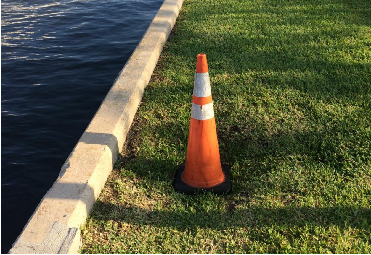
Figure 3.17: Sta 10+80. Area with backfill loss.
