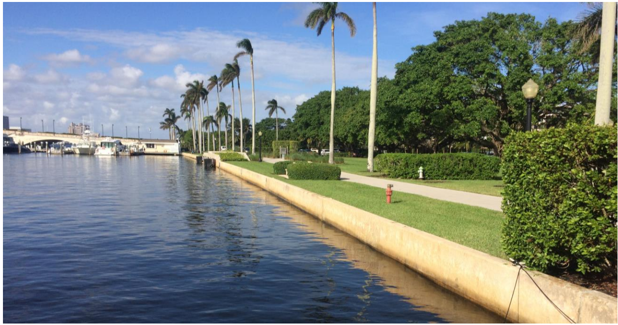
Figure 2.1: Sta 8+80 looking north. View of seaward face of the bulkhead at high tide.
