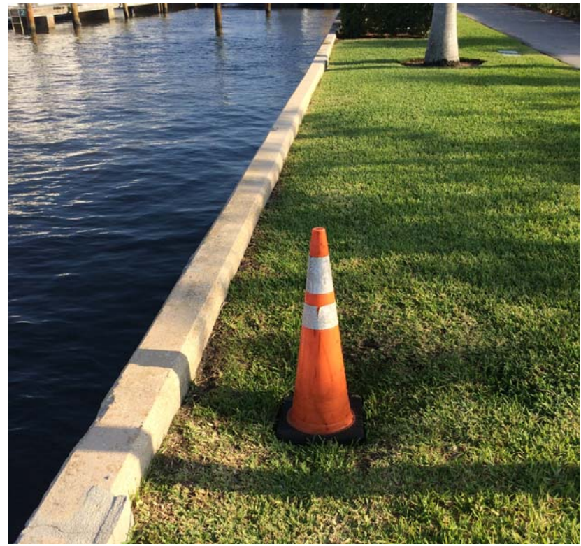
Figure 8.5: Backfill Loss behind the Bulkhead
