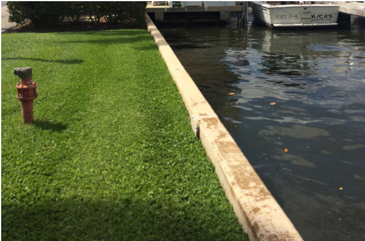
Figure 3.1: Sta 8+00 looking south. View of backfill close to the bulkhead cap elevation.
