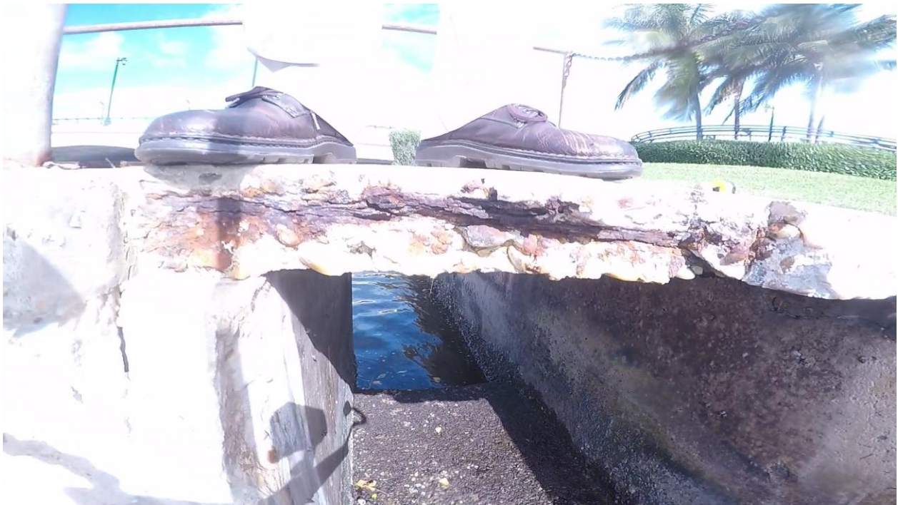
Figure 3.15: Sta 0+88 looking north. Spalling and rebar exposure and corrosion of the walkway to the outfall structure.
