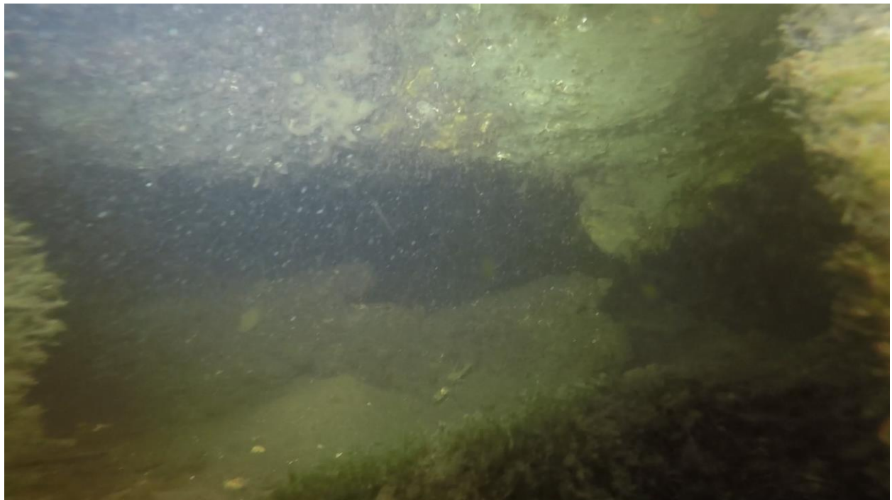
Figure 3.12: Sta 15+15. Gap underneath the corrugated section of the bulkhead and vague outline of a secondary sheet pile wall in the background.
