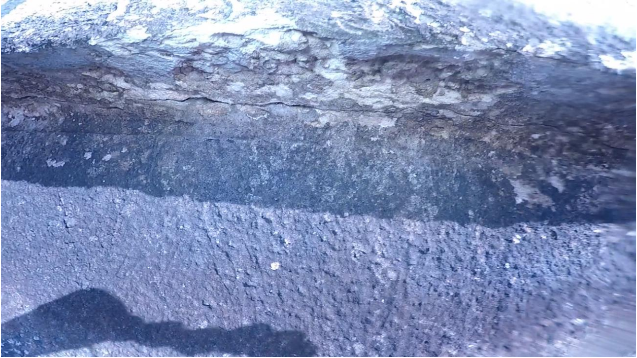
Figure 3.13: Sta 15+00. Cracking, spalling and deterioration underneath the lip along the parapet bulkhead section.
