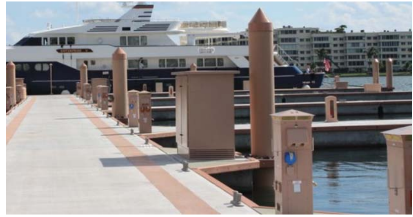
Figure 6.1: Typical Pedestal for Electrical, Water and Internet/Phone connection (Palm Harbor)
