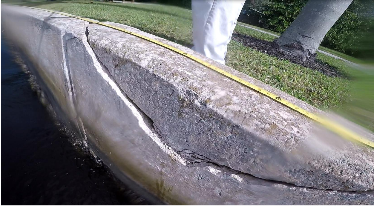
Figure 3.16: Sta 2+10. Crack and dislocated concrete cap.
