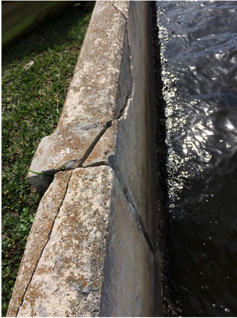
Figure 8.6: Cracking in the Bulkhead
