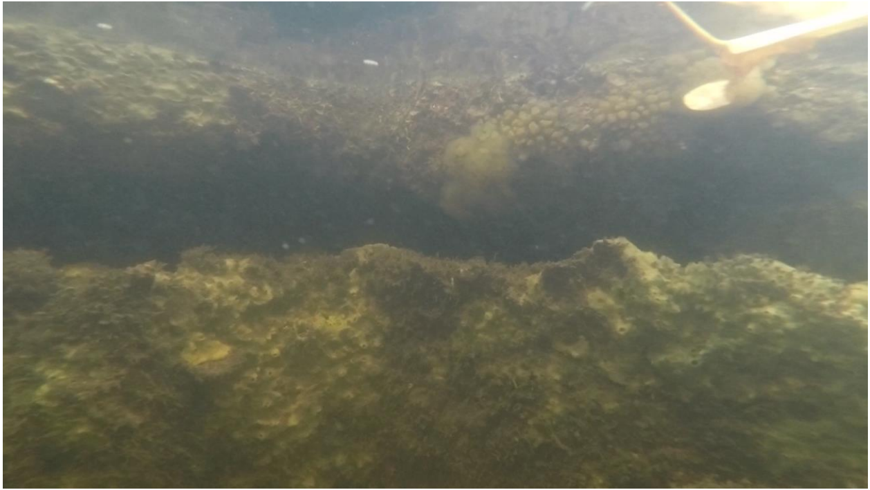
Figure 3.9: Sta 0+03. Horizontal cracks in the concrete bulkhead.
