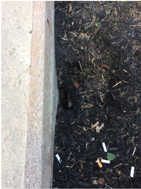
Figure 3.18: Sta 9+40. Area of backfill loss in front of Australian Dock office.
