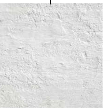
CAST STONE AND STUCCO TRIM SHERWIN WILLIAMS "BREAKERS OYSTER WHITE" CUSTOM COLOR (TO MATCH EXISTING)
