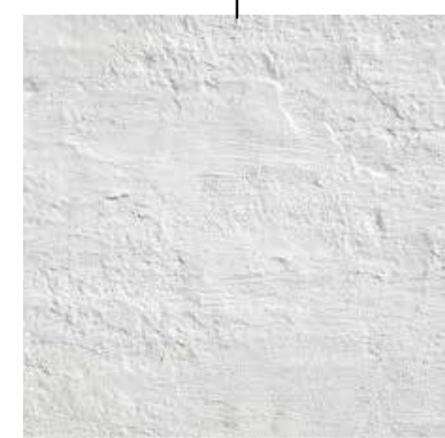
CAST STONE AND STUCCO TRIM SHERWIN WILLIAMS "BREAKERS OYSTER WHITE" CUSTOM COLOR (TO MATCH EXISTING)
