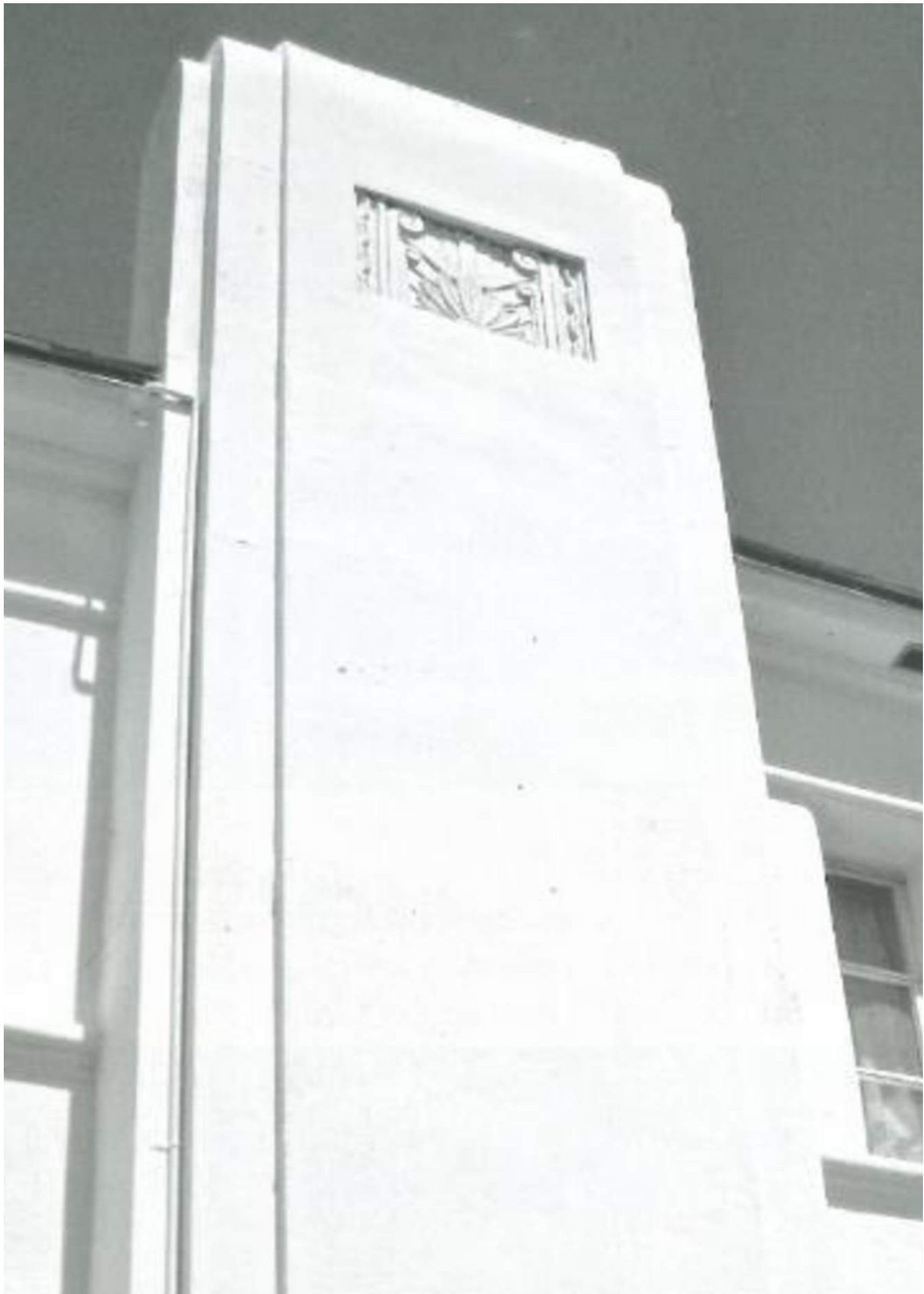
STUCCO WALL STEP, RELIEF DETAIL
