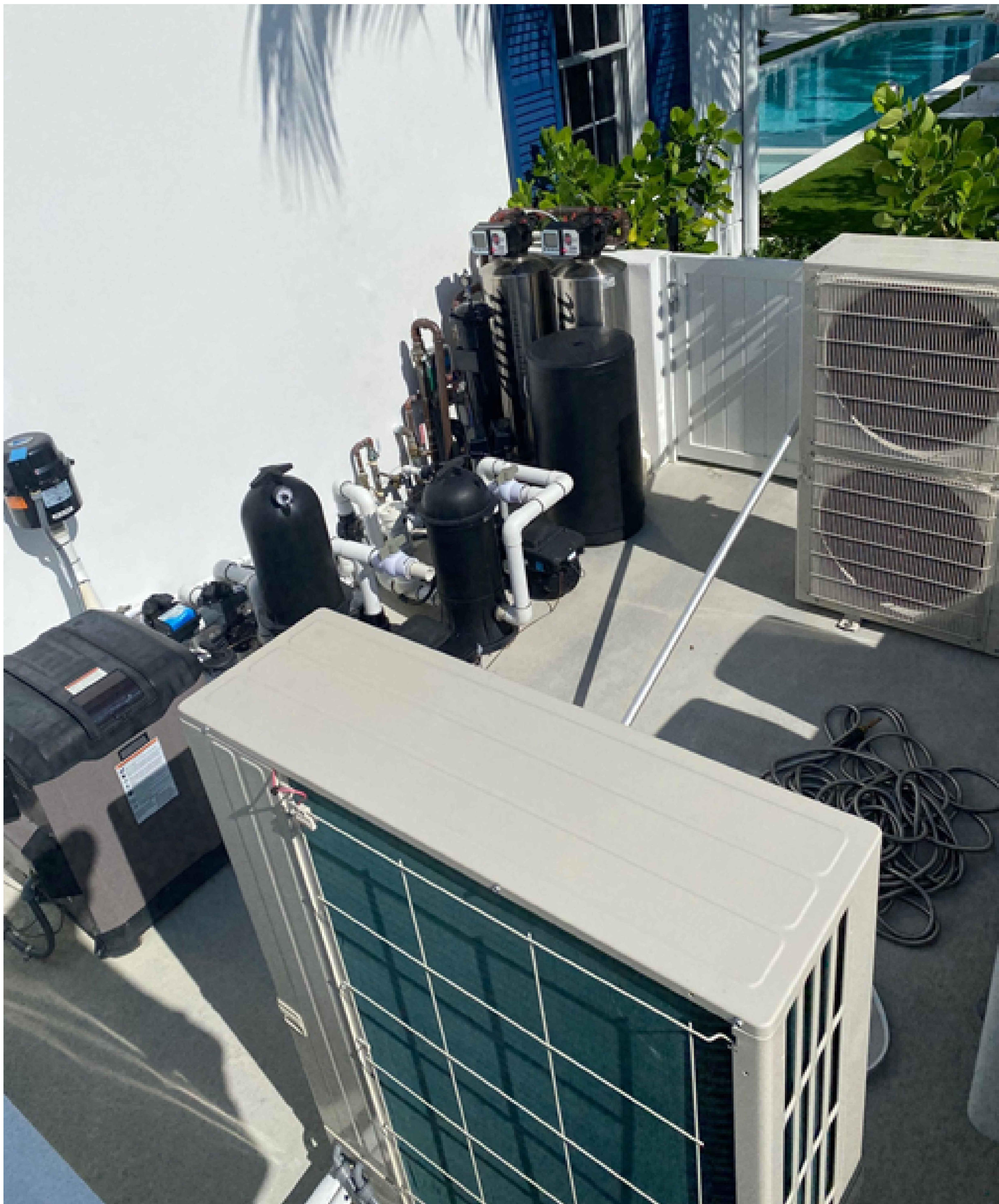
310 Clarke Avenue (Eastern Yard Equipment Area)
